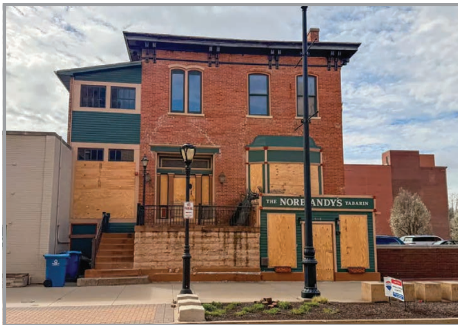
The property built by Virgil Hickox in 1839 at 518 E. Capitol Ave. was boarded after being damaged by a fire in February. PHOTO BY ZACH ADAMS
