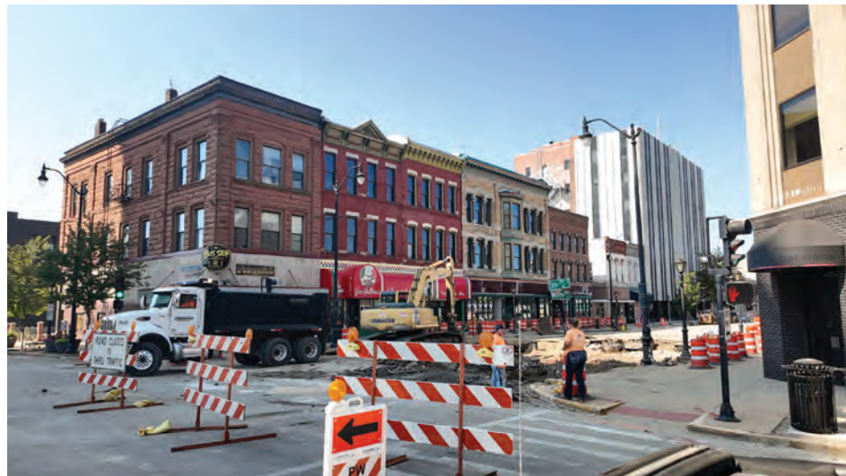
A 12-foot section of underground cast iron pipe burst Aug. 27 near the corner of Fifth and Monroe streets, flooding the street and causing damage to several nearby businesses. The Bus Stop, which was scheduled to have its grand opening the next day, suffered the majority of the damage, which isn't covered by insurance since the water came from an outside source. PHOTO BY ZACH ADAMS
