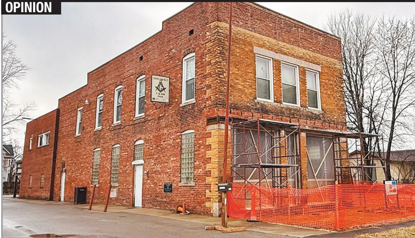
New large mahogany doors and all-yellow brickwork on the façade of the Black Firehouse at 1310 E. Adams St. are the latest renovations expected to be completed by the end of August on this historic structure. The building, owned by the Central Lodge #3 Prince Hall Masons, was the first Black firehouse in Springfield. PHOTO BY ZACH ADAMS
