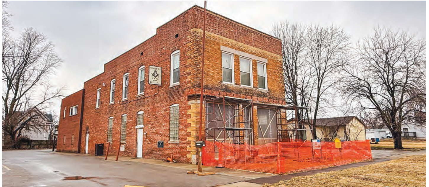
The former Black Firehouse at 1310 E. Adams St. is in the process of getting new mahogany doors and an updated façade. PHOTO BY ZACH ADAMS
