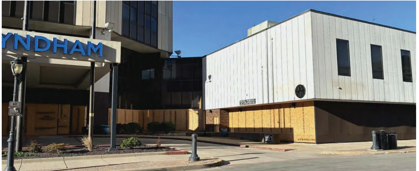
The Wyndham Springfield City Centre Hotel has been closed since March 27, 2025, when it was damaged by internal flooding. PHOTO BY JAMES BENGFORT
