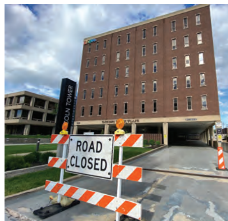
The ground-level and below-ground parking at the Lincoln Tower Apartments complex has been unavailable for use since February 2023 when the city decided the deteriorating parking areas were unsafe. The parking was also used by tenants of Lincoln Tower Plaza, an office building immediately west of the apartment complex along South Second Street in Springfield. PHOTO BY DEAN OLSEN
