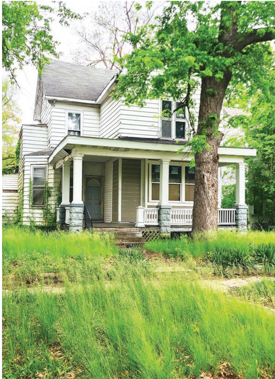
The house at 820 N. Sixth St. on April 29, the day George Petrilli transferred the property back to Enos Park Development. The house has remained uninhabitable since he originally acquired the property from the nonprofit 12 years ago and became a source of controversy during last year's mayoral election. PHOTO BY MICHELLE OWNBEY.
