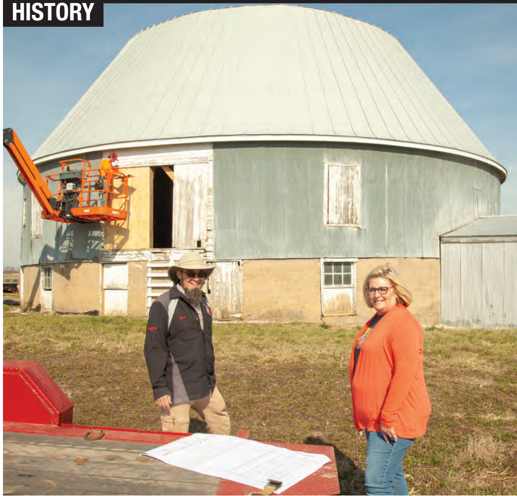
Contractor Glenn Beechy, left, and Laura Pickrell review plans for renovations of the round barn.
